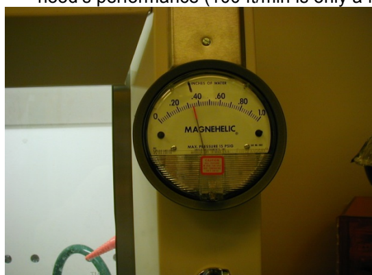
*“Magnehelic gauge” – note normal gauge position. Significant deviation may indicate low air flow.
